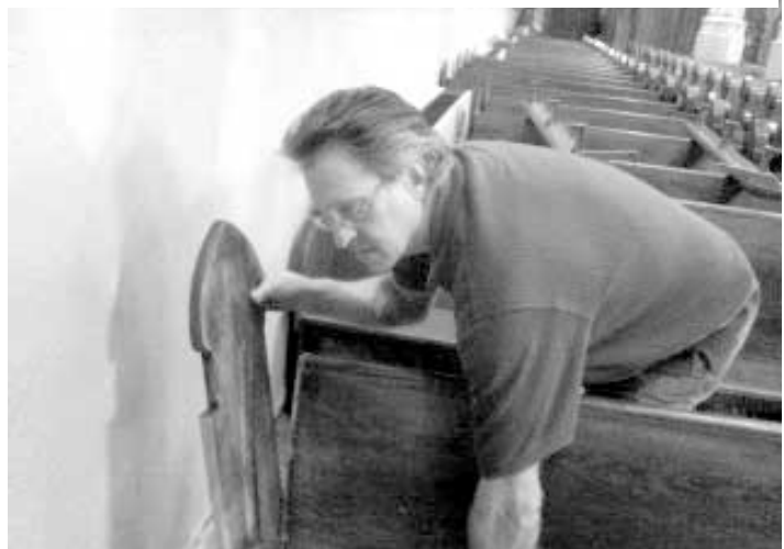
Parishioner Bob Molinski works on fixing the pews at the side entrance. One of the pews had broken, so it is being reworked into a pamphlet rack. The space between pews was enlarged to provide for those with wheelchairs or walkers.
