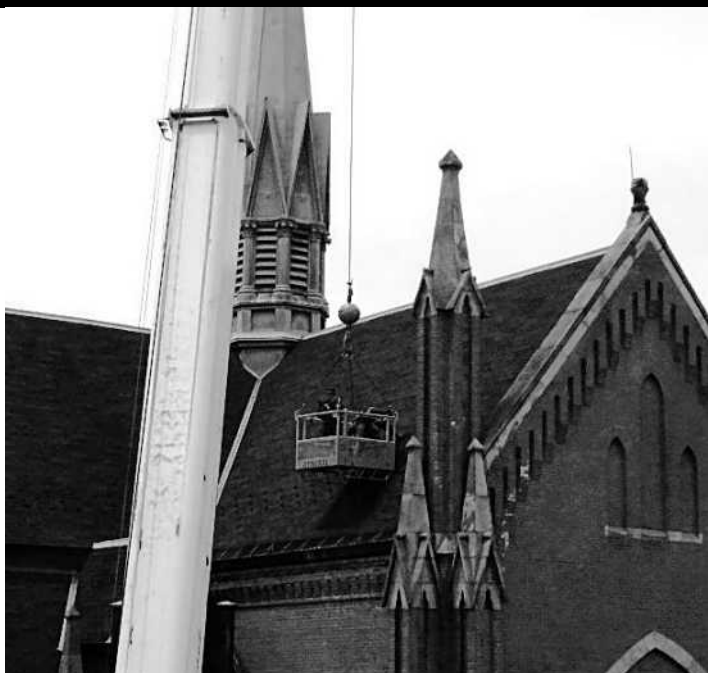
Last week we had major repair work done on three roofs. Because the damage was from storms, insurance covered the cost, minus a $1,000 deductible paid by the parish. By keeping up with repairs, we have been able to extend the life of the roof much longer than anticipated.
