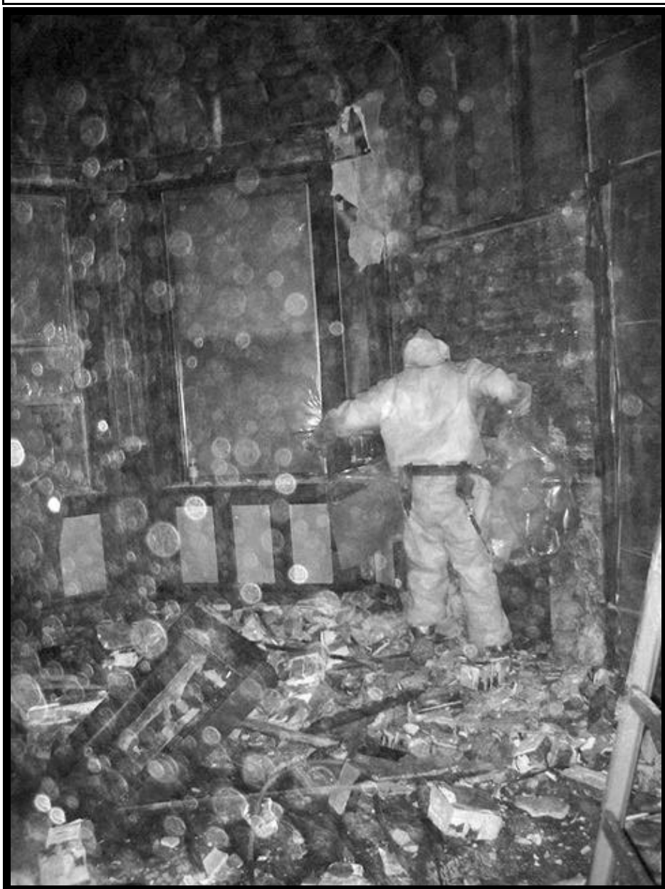
Worker in protective suit removing asbestos material from the rectory living room
