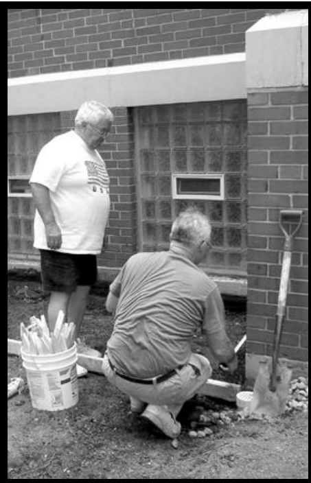
Joe Calamante and Patrick Racut prepared the forms for the concrete walks in the rectory gardens.
